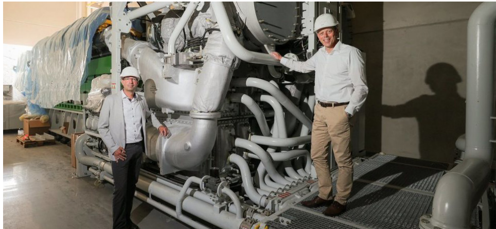
Engineering Director Michael Berger (right) and Sales Manager Sebastian Pongratz from Fernwärme Ulm next to the new Jenbacher J920 Flextra
